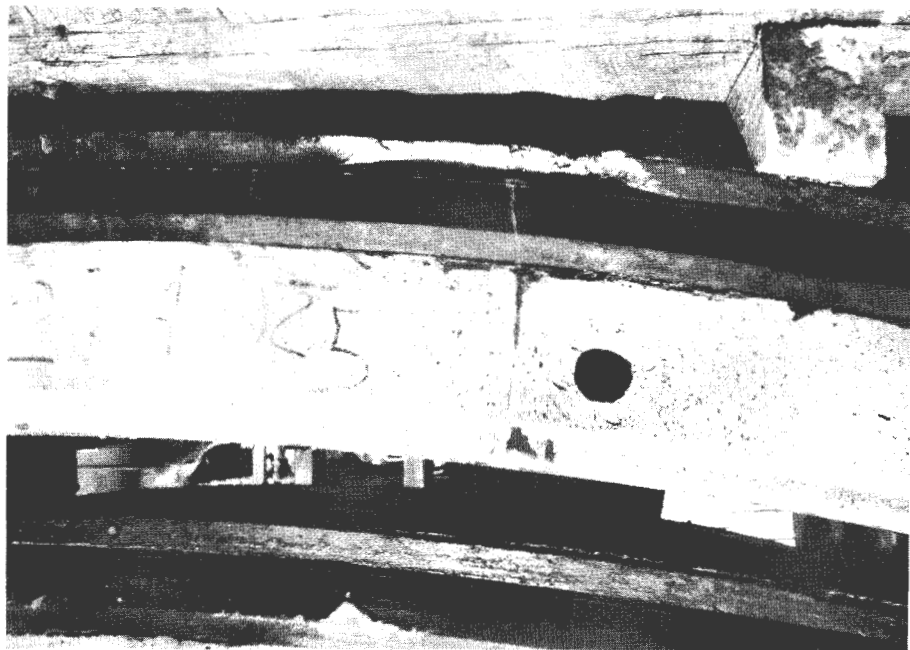
FIGURE 126. DAMAGE CAUSED BY FORKLIFT
