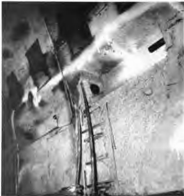
FIGURE 132. EXPOSED REBAR IN RING #450.
