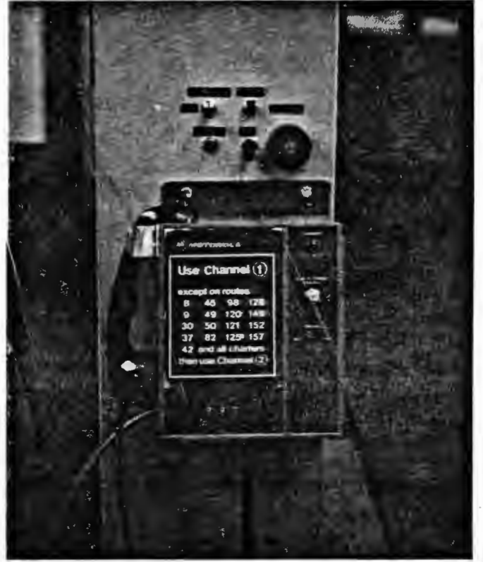
On-Vehicle communication equipment set up at the CTA control center for training staff. (Chicago)
