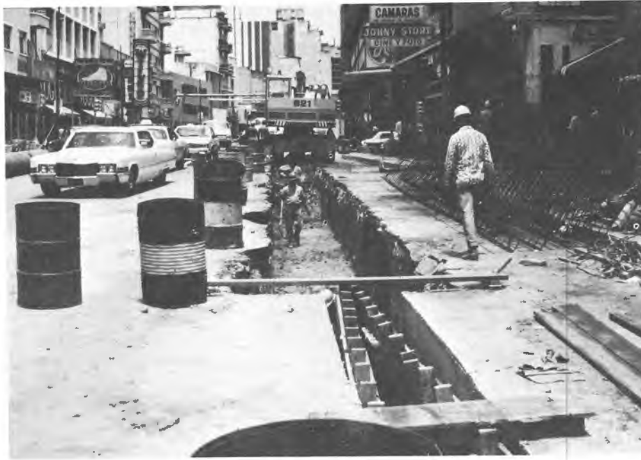
(a) Traffic Maintained Through Construction Site where Guide Walls are Being Made
