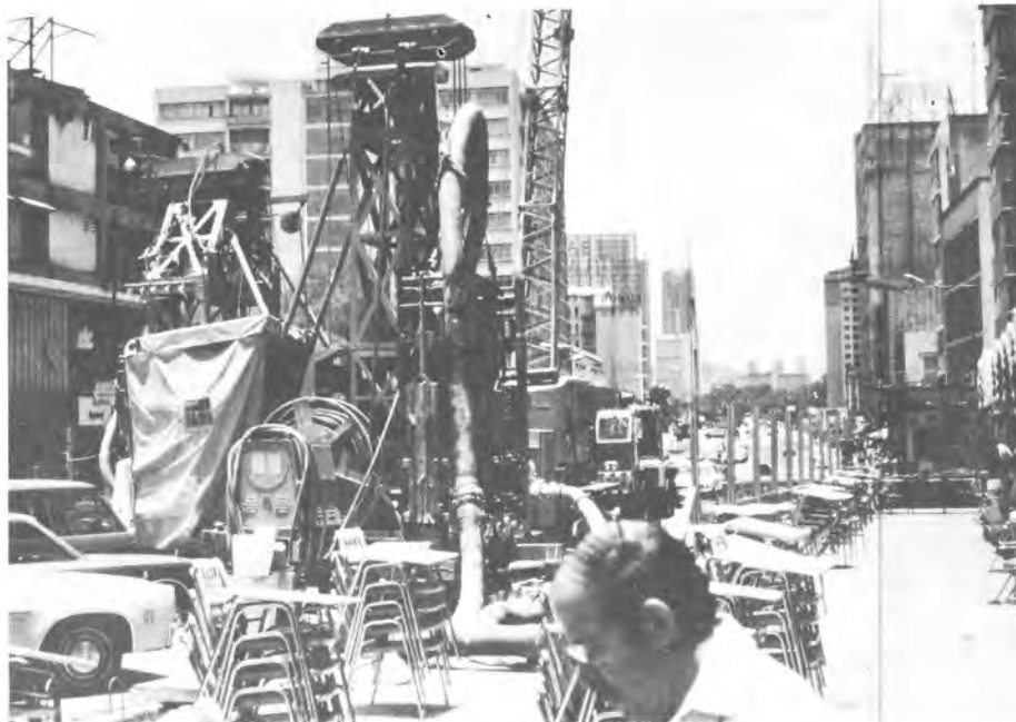
(b) Slurry Wall Trenching Machine Operating Adjacent to Sidewalk Cafe. Open for Business.
