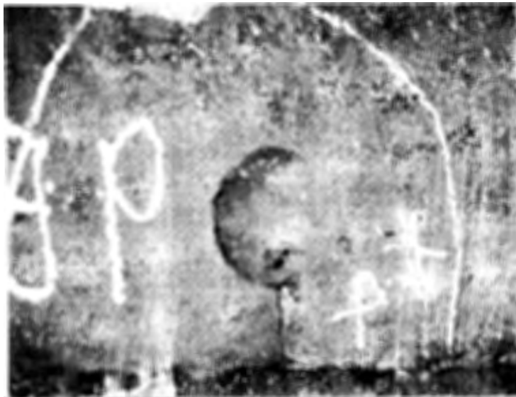
Obvious Cracking at a Rivet Hole
