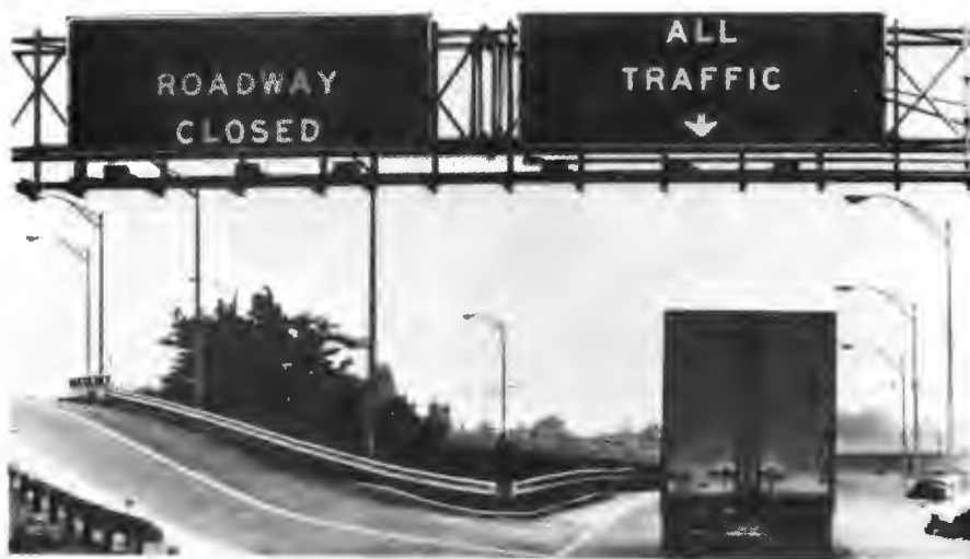
Figure 2-9. Rotating Drum Signs on the New Jersey Turnpike
