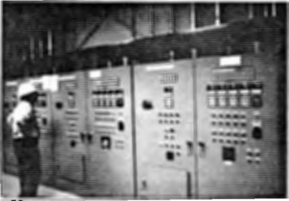
Continuous record of furnace temperature.
