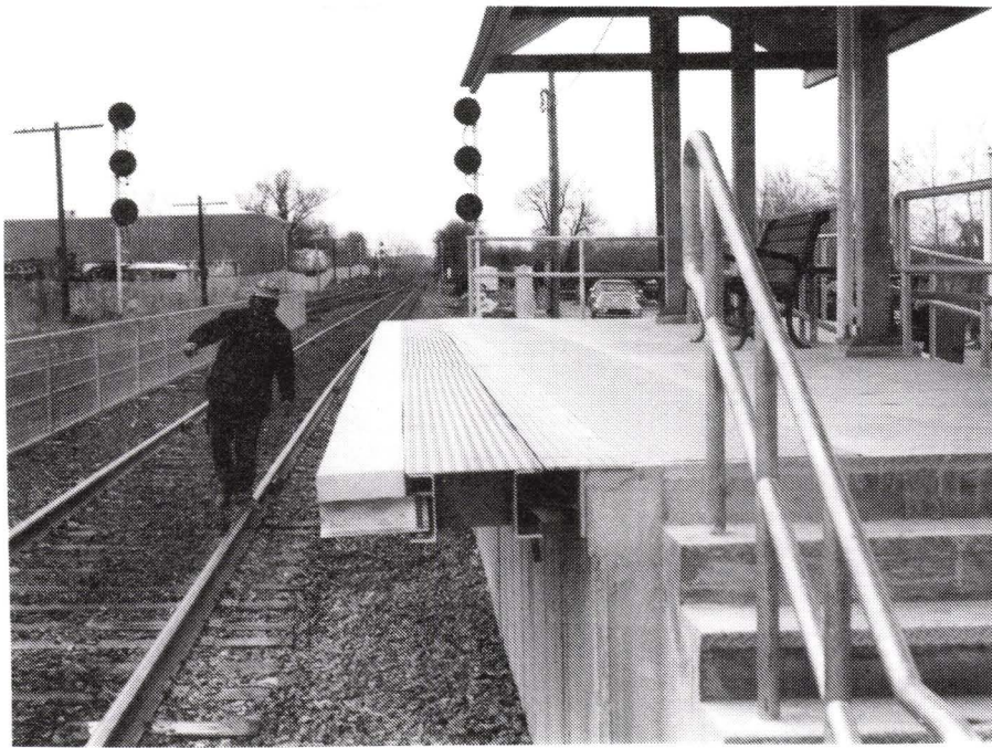
FIGURE 4-2 FRANGIBLE ← PLATFORM EDGE AT MBTA MISHAWUM STATION (DEPLOYED)
