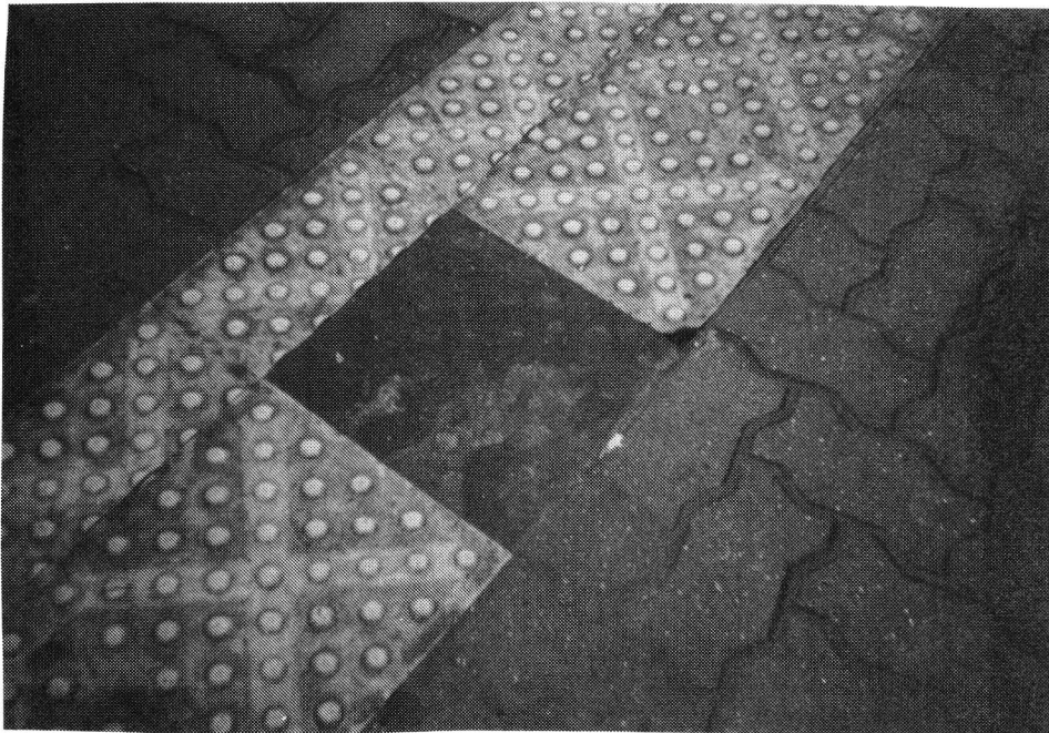
FIGURE 3-3. TILE LIFT-OFF SACRAMENTO MALL
