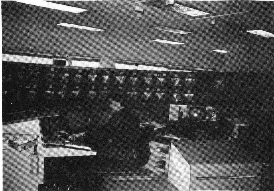
FIGURE 3-19. CLOSED CIRCUIT TV SURVEILLANCE (VANCOUVER SKYTRAIN)
