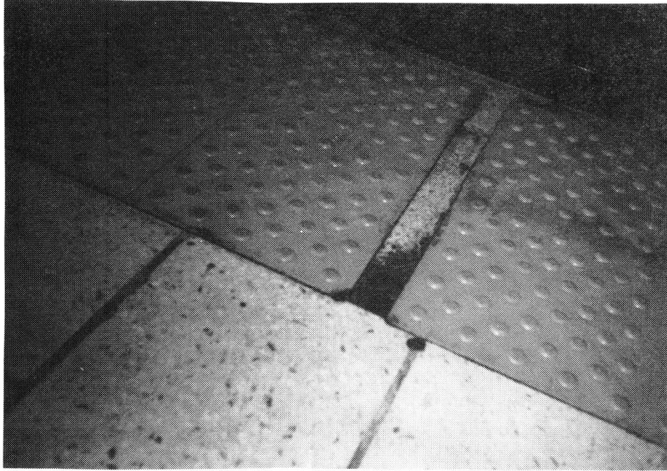
FIGURE 3-2. TILE LIFT-OFF LAKE MERRITT STATION
