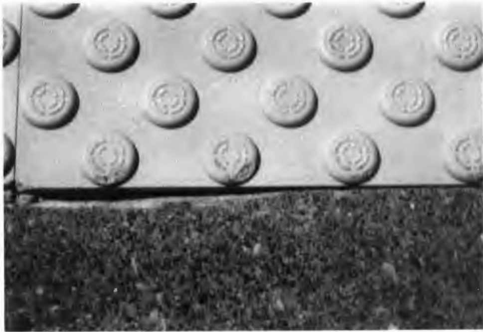
Figure 3-5 Transpo Industries: Step-Safe Installation at GCRTA Triskett Street Station Illustrating Chipped Domes (Photo Taken After 200 Exposure Days)
