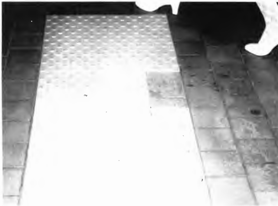
Figure 3-2 Rehau: Access Tactile Tile Installation at MBTA South Station Illustrating Missing Tile (Photo Taken after 78 Exposure Days)
