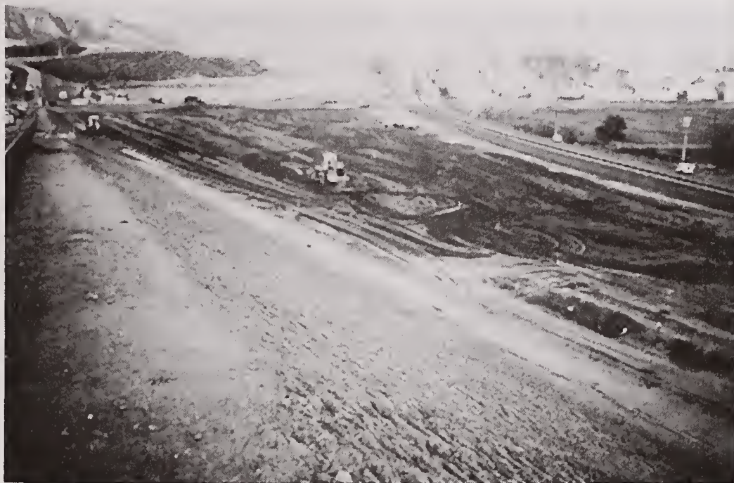
Parking lot of the new Princessa/ Canyon Country Station on the Santa Clarita Line being graded.
