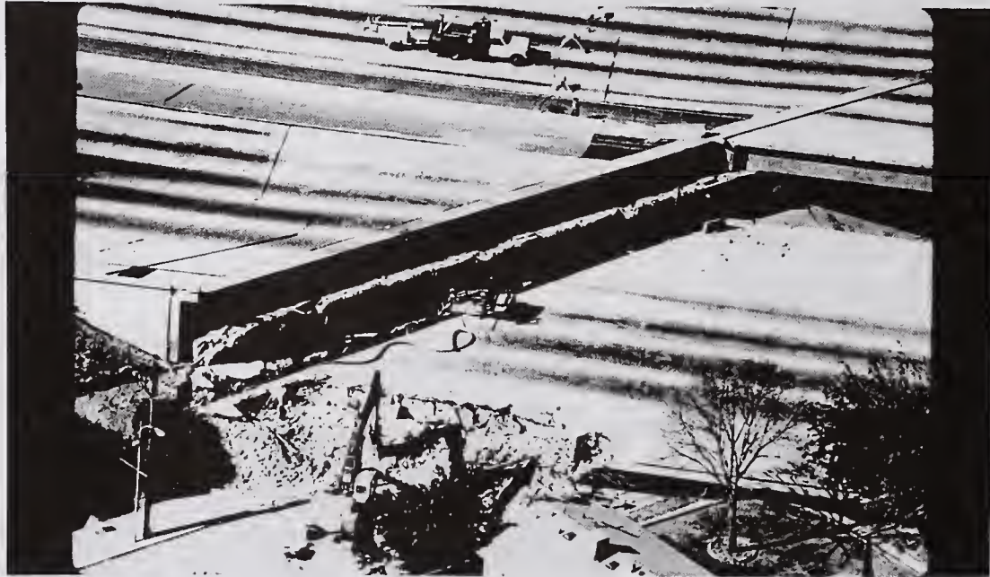
State Route 118 (Simi Valley Freeway). Detour at Woodley Avenue west of the State Route 405 (San Diego Freeway).
