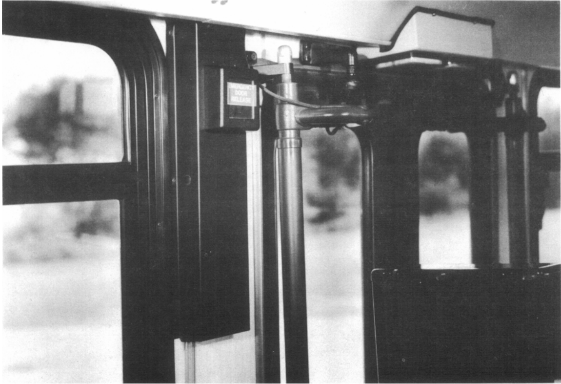
PHOTOGRAPH 2-48 NEOPLAN USA MODEL: REAR DOOR BOX CONTAINING EMERGENCY DUMP VALVE
