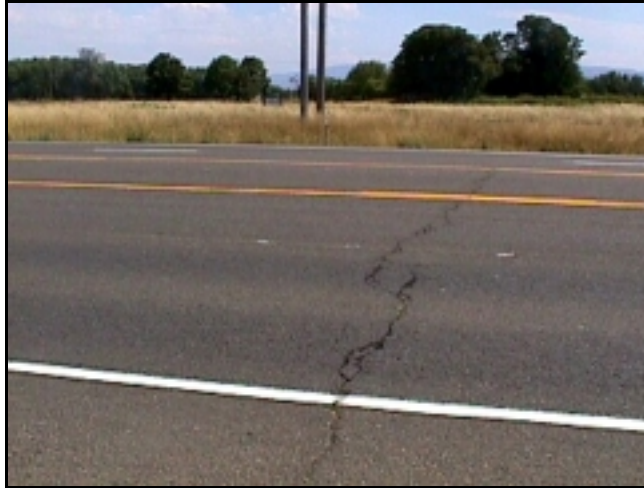
Figure 4.23: Transverse Crack on ORE 99 at MP 111.5 SB
