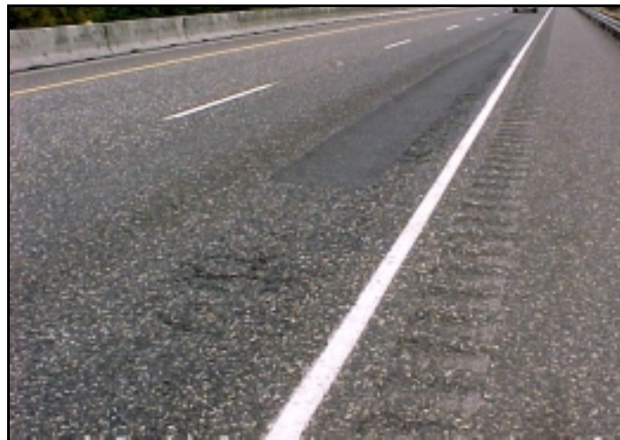
Figure 4.14: Distressed and Patched F-mix at MP 28.6 WB, Looking West, September 2001
