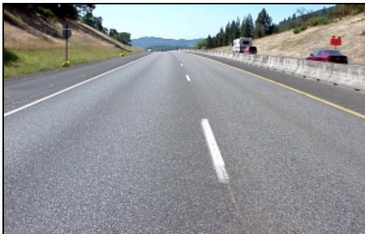
Figure 4.32: Full-width, 1.6 Km (approx.) Inlay of Outside Lane with F-mix, I-5 NB in Roseburg
