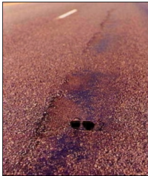
Figure 3.14: Close-up Image of I-84 Stripping, 1997
