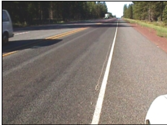
Figure 4.33: Stud Rutting on US 97 near Bend at MP 150.2 SB, July 1999, Prior to Repair
