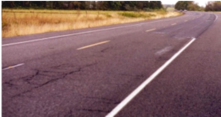
Figure 4.15: 1997 Distress and Screed Patch on ORE 99W near MP 77 NB
