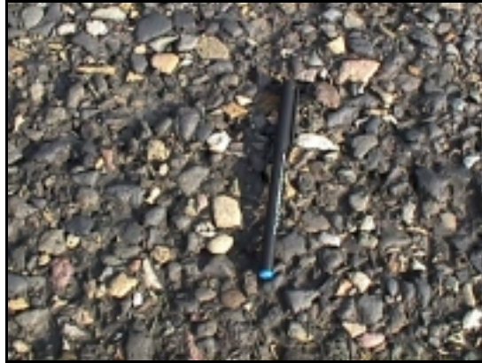
Figure 4.11: I-84, MP28 WB, Aggregate Loss in Outside Wheelpath, August 1999
