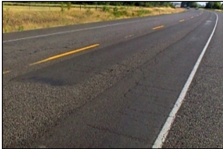
Figure 4.18: Two-year Old Screed Patches at Same Location as Figure 4.17, 1999
