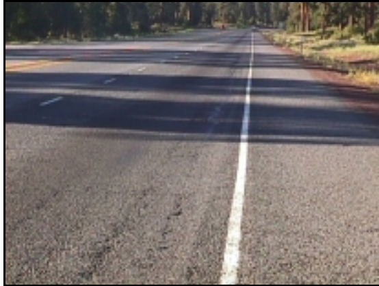
Figure 4.39: F-mix Distress at MP 148.4 SB prior to July 1999 Repair
