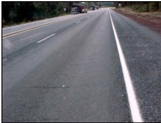
Figure 4.40: MP 148.4 SB Condition after Two Years
