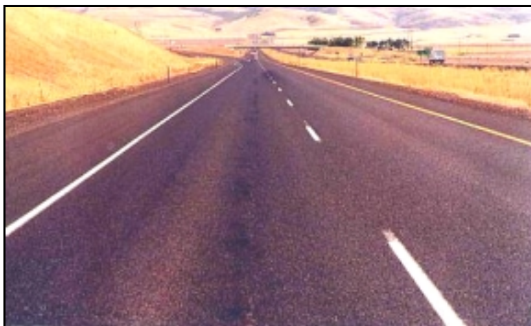
Figure 3.15: Stripping at MP ~215.5, I-84 WB Lanes near Pendleton, Looking East, July 1997
