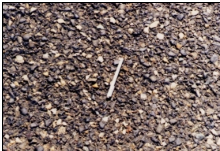
Figure 4.10: I-84, MP28 WB, Aggregate Loss in Outside Wheelpath, August 1997
