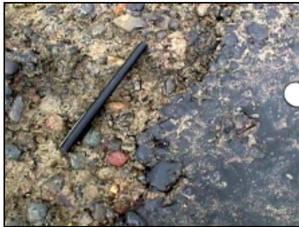
Figure 3.13: Close-up of Distress of Figure 3.12
