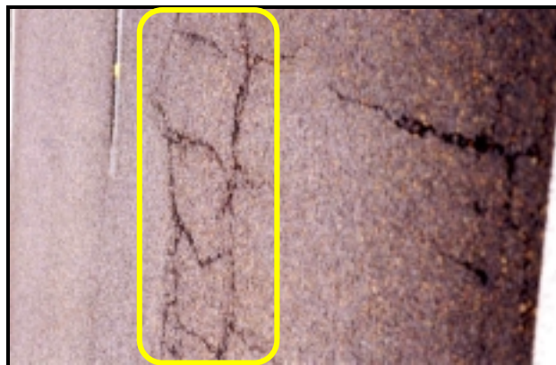
Figure 4.16: Close-up of Distress from Figure 4.15
