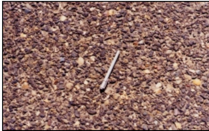
Figure 4.12: I-84, MP28 WB, Aggregate Retention on Shoulder, August 1997
