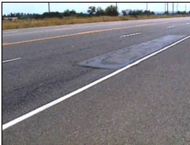
Figure 4.25: Cracks and Patching on ORE 99 at MP 112.8 SB
