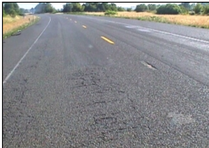
Figure 3.8: Alligator Cracking on ORE 99W North of Corvallis, 1999, prior to Resurfacing
