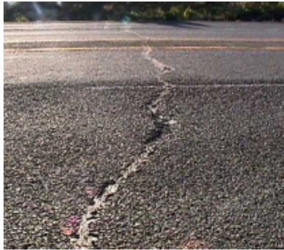
Figure 3.18: Thermal Cracking on US 97, ~MP 149, near Bend
