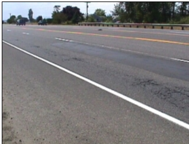
Figure 4.27: Crack and Patch on ORE 99 at MP 112.2 NB
