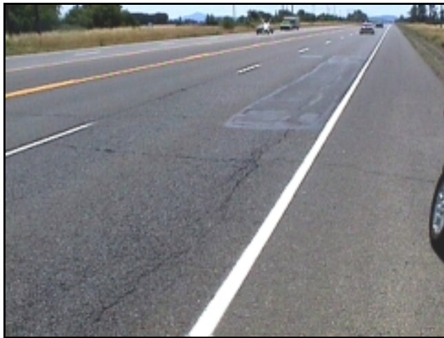
Figure 4.24: Cracks and Patching on ORE 99 at MP 111.8 SB
