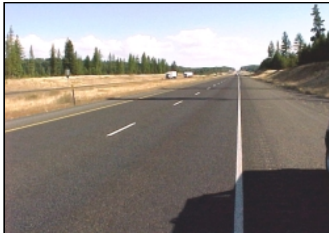
Figure 4.3: Pavement Surface near MP 238 EB, September 2001, Four Years after Fog Seal
