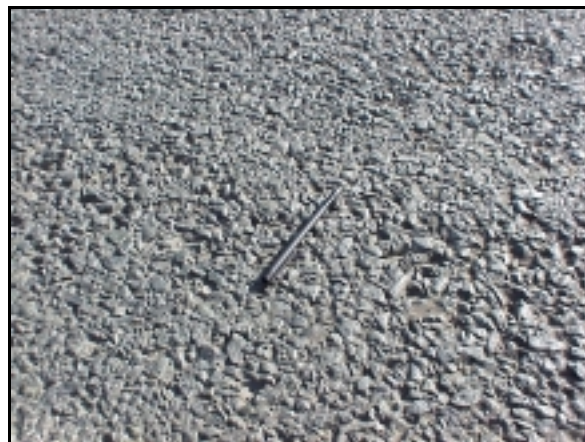
Figure 3.4: Close-up of Wheeltrack Pavement Surface, ORE 42, MP 18 (approx.)
