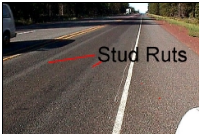
Figure 3.1: Stud Rutting on US 97, MP 150.2 SB near Bend
