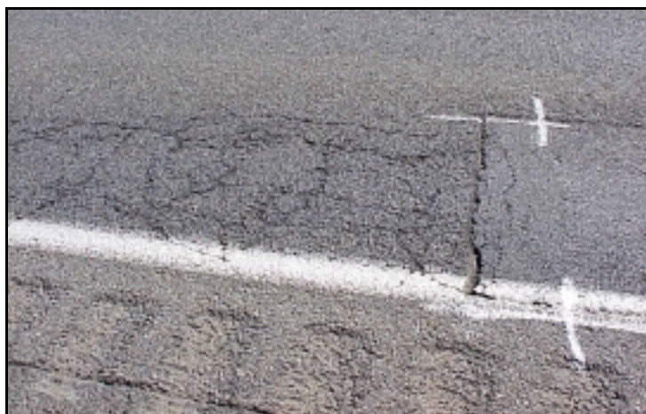
Figure 4.30: Distress at North Edge of Figure 4.28 Plug Patch, which Occurred after Patch was Installed
