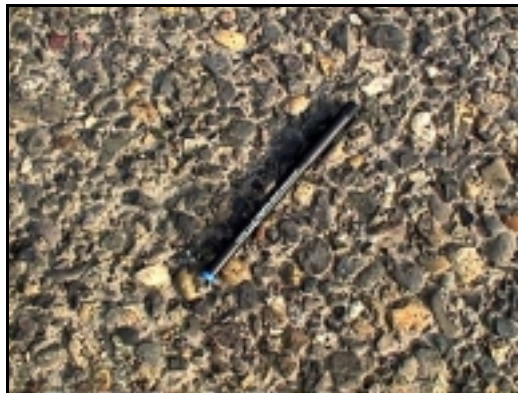
Figure 4.13: I-84, MP28 WB, Aggregate Retention on Shoulder, August 1999
