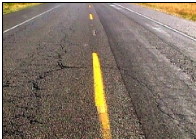
Figure 4.19: Close-up of Two-year Old Screed Patches Compared to Non-patched SB Lane
