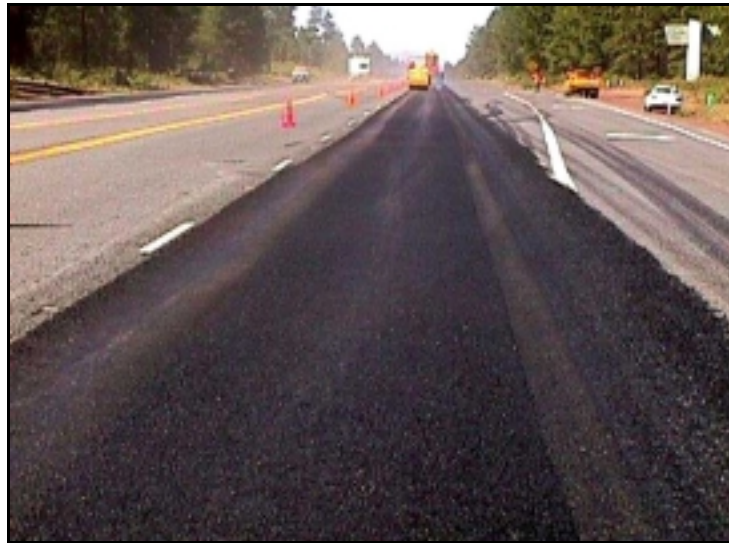
Figure 4.38: Outside Lane Repair and Unrepaired Passing Lane, US 97 approx. MP 149.5 SB, July 1999
