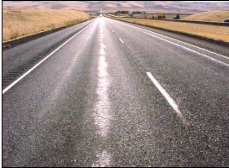
Figure 3.16: Stripping on I-84, ~MP 215.5 WB Lanes, Looking East, September 2001
