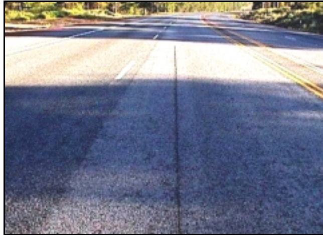
Figure 3.2: Gouging on US 97 near Bend
