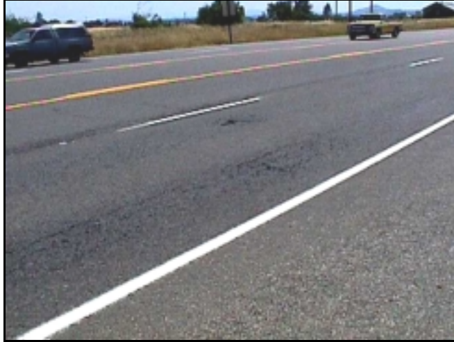
Figure 4.26: Raveling on ORE 99 at MP 114.1 SB
