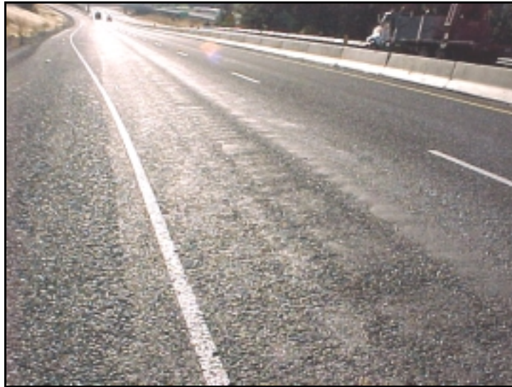
Figure 4.6: Tire Chain Damage, WB Lanes Looking East, near MP 252.6, September 2001
