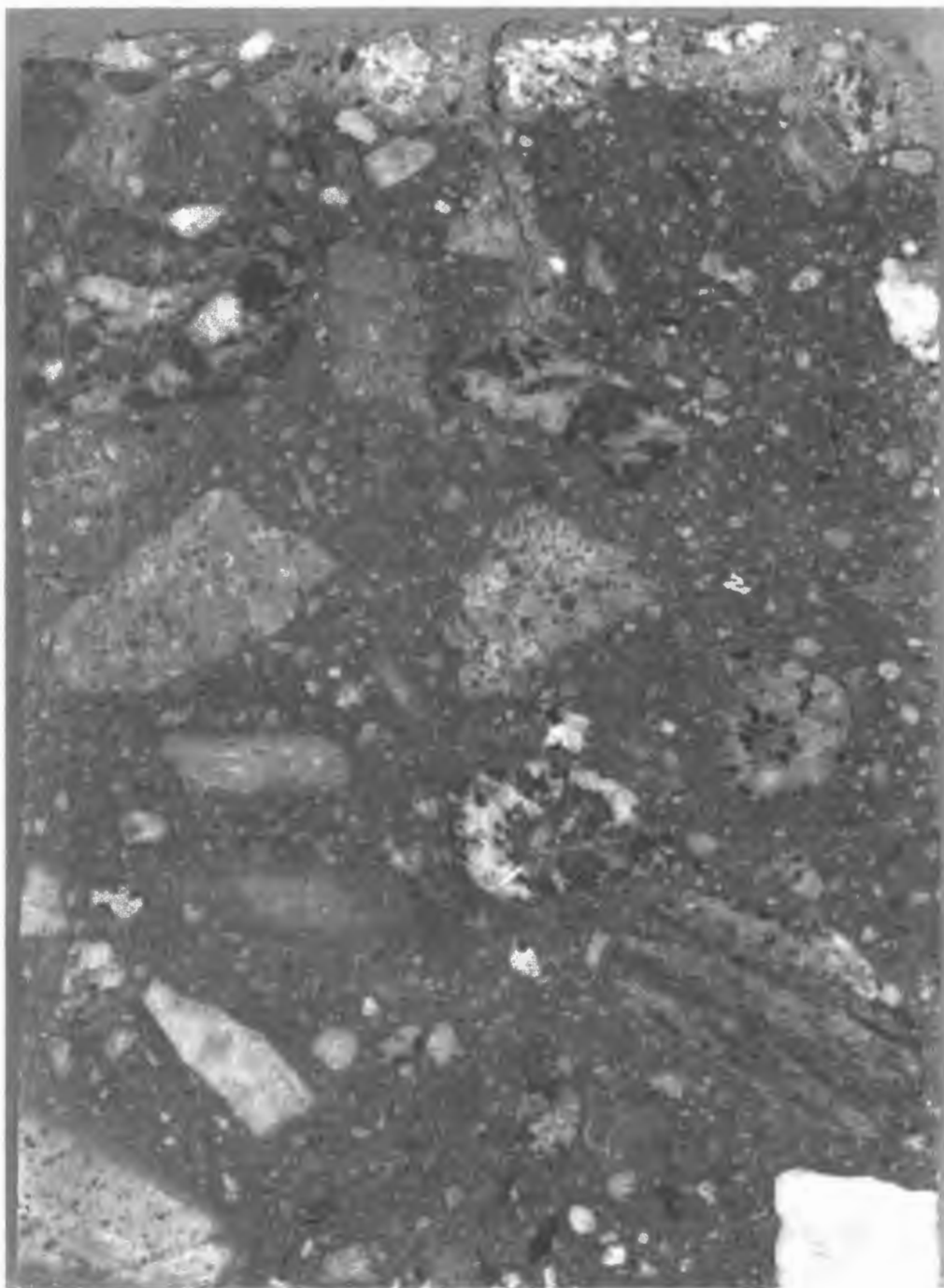
Figure 3-79. Phenolphthalein stained polished slab, showing carbonation along plastic shrinkage crack (magnified 1.5x).
