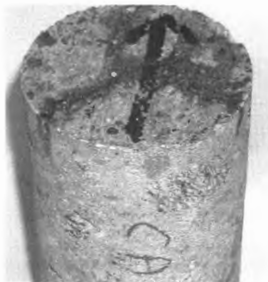
Figure 3-75. Map cracking pattern on core CA-014-011-001E, emphasized by wetting down the surface.
