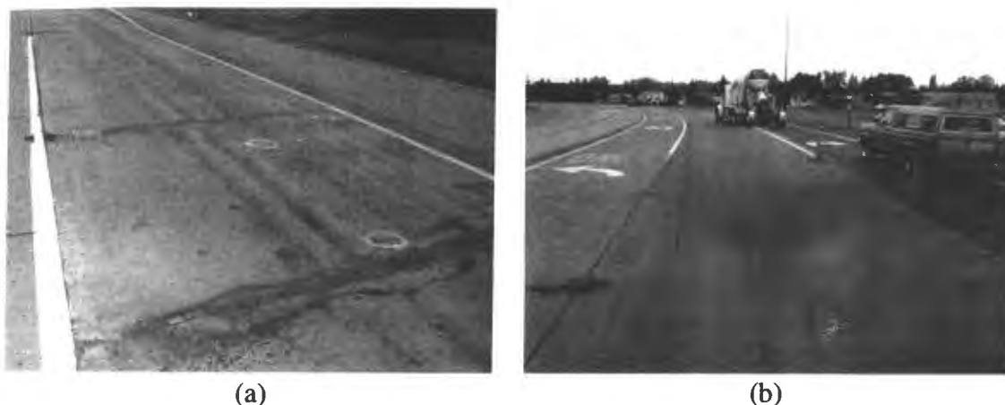
Figure 3-21. Typical distress manifestations observed at MN-065-064.
