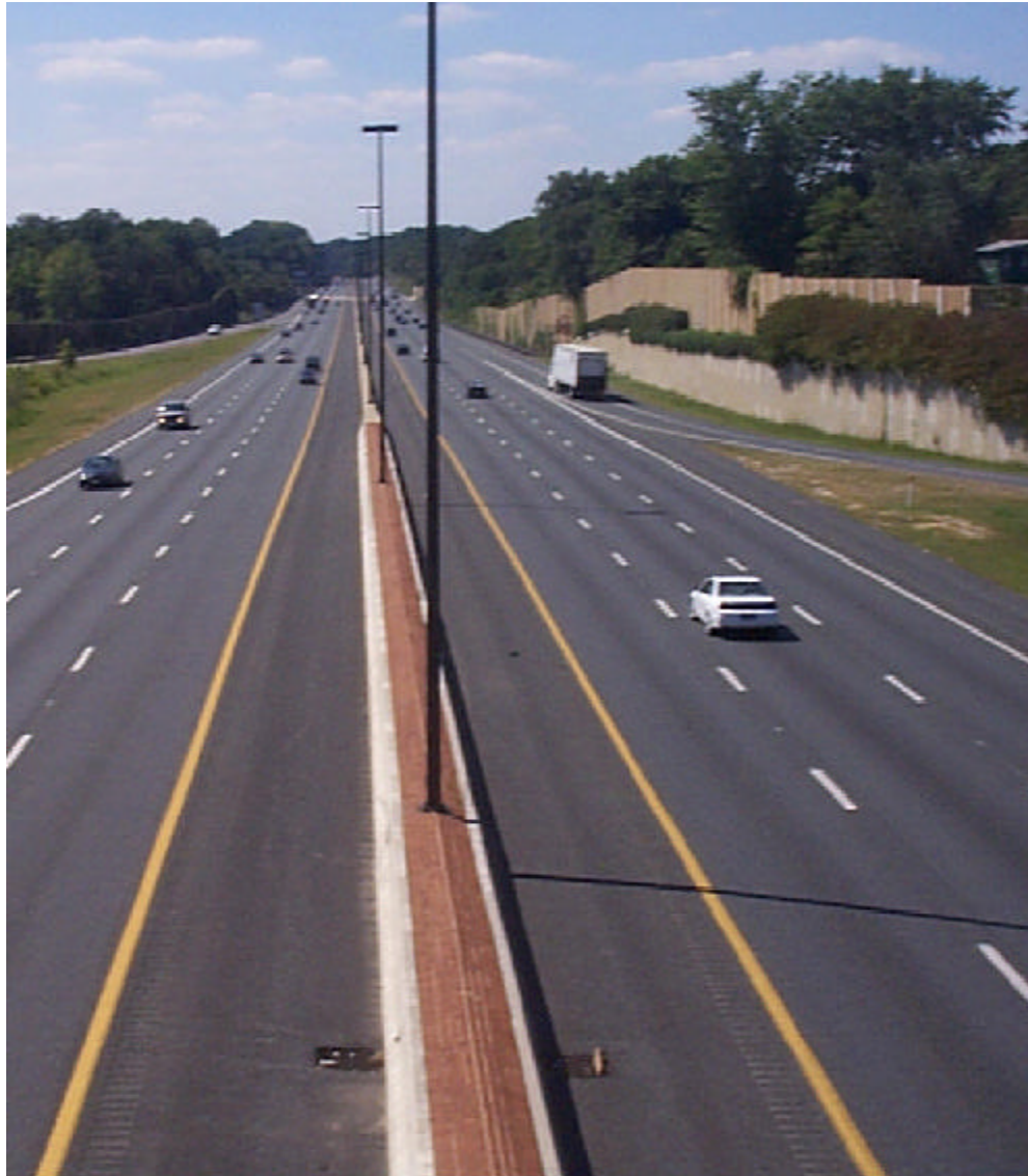
Heavy-duty stone matrix asphalt, first used in Europe, is now the top pavement choice for heavily traveled U.S. highways.
