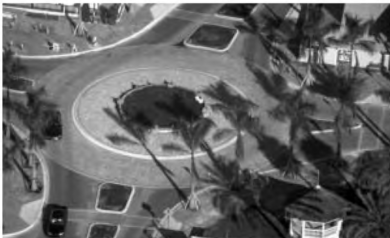
This Fort Pierce, Florida, roundabout is being constructed to reduce speeding, improve safety, and enhance the aesthetics of the community.
