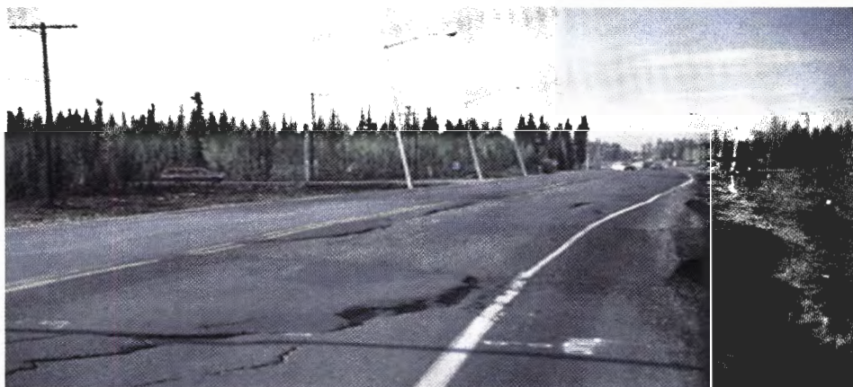
Figure 1. Photo of settlement and cracks on an Alaskan roadway due to warming of the permafrost foundation.
