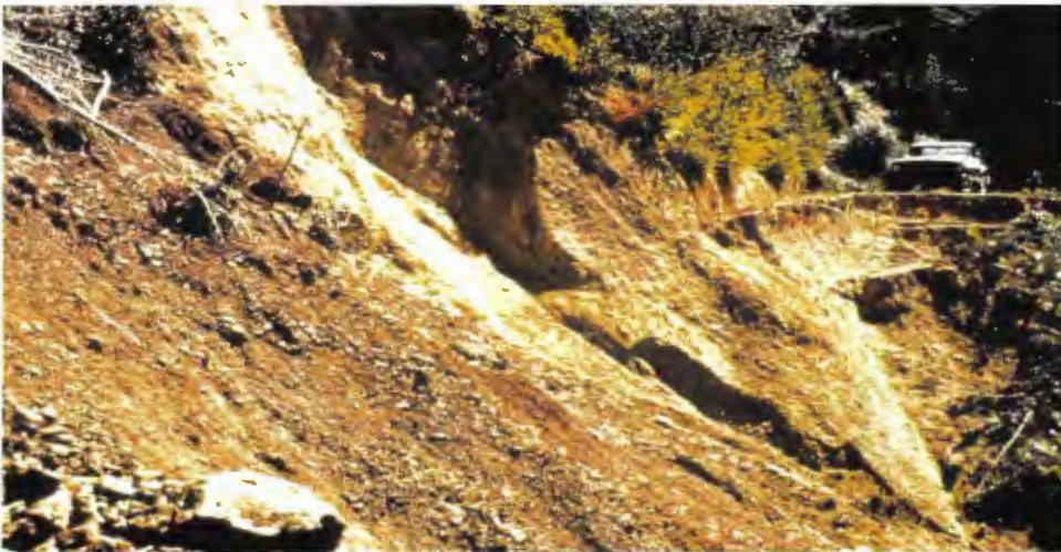
Figure 1. Photo of a roadcut failure. Cut banks on rural roads are often very close to vertical. These banks are more prone to failure as warmer more intense winter storms increase proportion of rain versus snow. Access to rural locations will be lost more frequently and roadway maintenance costs will rise.
