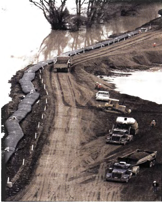
Figure 2. Photo of a levee breach in the Sutter Bypass. A warm winter storm in January 1997 caused this breach. A temporary bladder seen at left in the photo was used to protect the repair and prevent additional flooding from rising water levels in the bypass.
