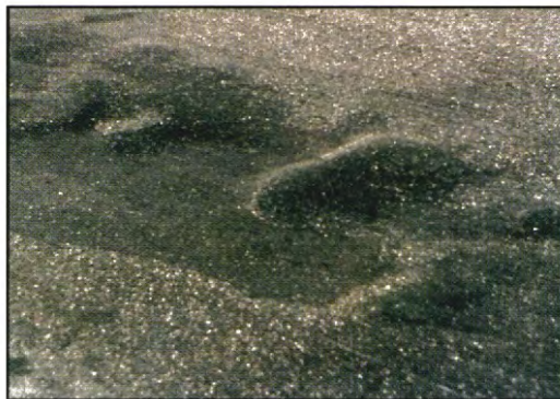
FIGURE 35 Distress Type ACP 10—Shoving in Pavement Surface
