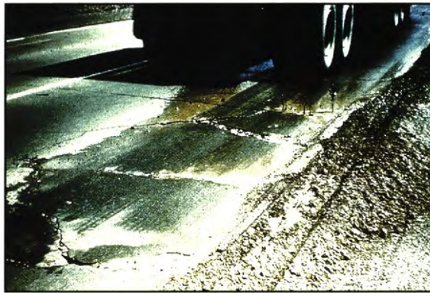
FIGURE 89 Distress Type JCP 16—Water Bleeding and Pumping
