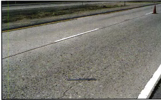
FIGURE 55 Distress Type JCP 3—Low Severity Longitudinal Cracking
