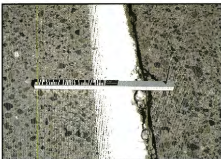
FIGURE 64 Distress Type JCP 6—Low Severity Spalling of Longitudinal Joint
