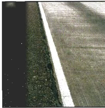
FIGURE 83 Distress Type JCP 14—Well-Sealed Lane-to-Shoulder Separation
