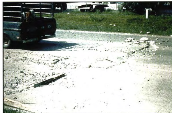
FIGURE 76 Distress Type JCP 11—A Blowup
