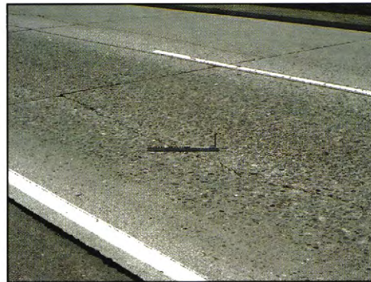
FIGURE 56 Distress Type JCP 3—Moderate Severity Longitudinal Cracking
