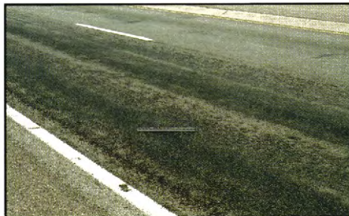
FIGURE 37 Distress Type ACP 11—Loss of Texture
