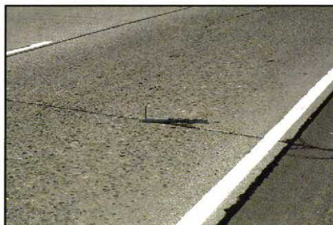
FIGURE 67 Distress Type JCP 7—Moderate Severity Spalling of Transverse Joint, Far View
