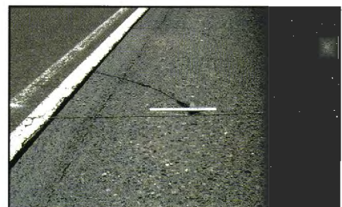
FIGURE 50 Distress Type JCP 1—Moderate Severity Corner Break
