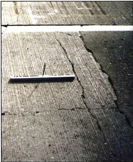
FIGURE 125 Distress Type CRCP 12—Moderate Severity Punchout
