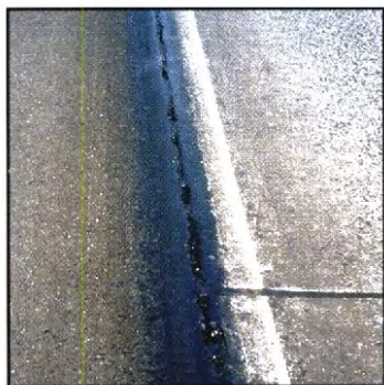
FIGURE 82 Distress Type JCP 14—Poorly Sealed Lane-to-Shoulder Separation
