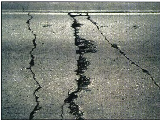
FIGURE 100 Distress Type CRCP 3—High Severity Transverse Cracking
