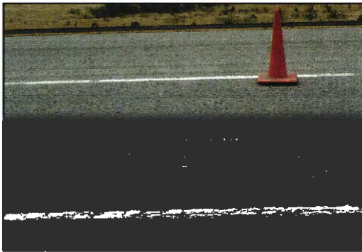
FIGURE 98 Distress Type CRCP 3—Low Severity Transverse Cracking
