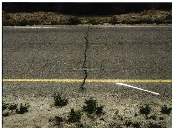
FIGURE 21 Distress Type ACP 6—High Severity Transverse Cracking
