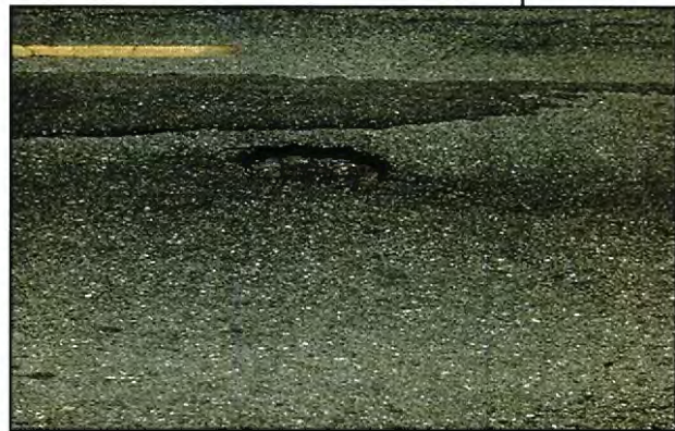
FIGURE 28 Distress Type ACP 8—Moderate Severity Pothole
