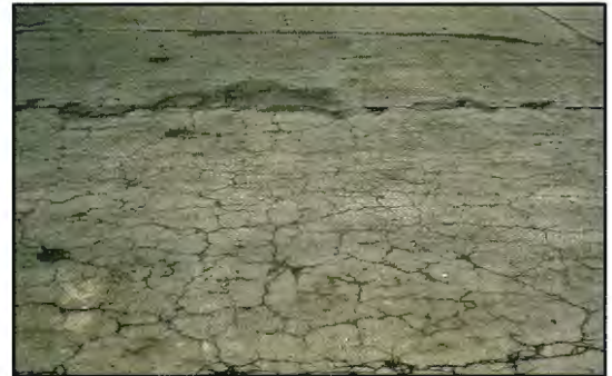
FIGURE 69 Distress Type JCP 8a—Map Cracking
