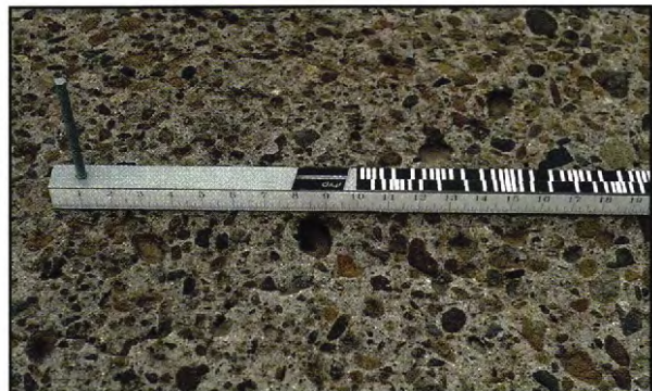
FIGURE 105 Distress Type CRCP 6—Popouts
