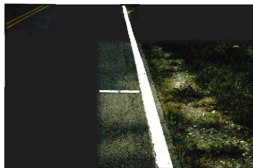
FIGURE 12 Distress Type ACP 3—Low Severity Edge Cracking
