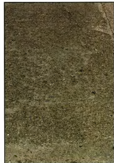
FIGURE 102 Distress Type CRCP 4b—Scaling
