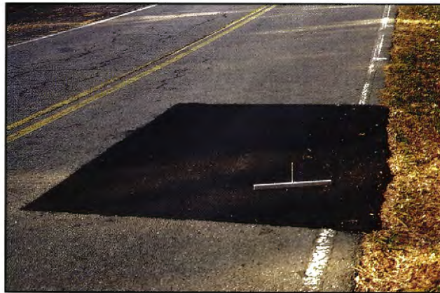
FIGURE 24 Distress Type ACP 7—Moderate Severity Patch
