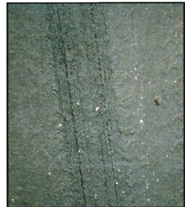
FIGURE 38 Distress Type ACP 11— Aggregate Obscured
