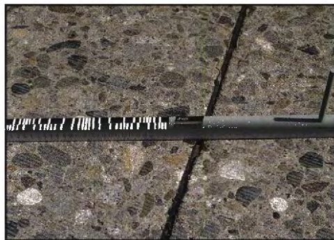
FIGURE 133 Distress Type CRCP 15—Longitudinal Joint Seal Damage
