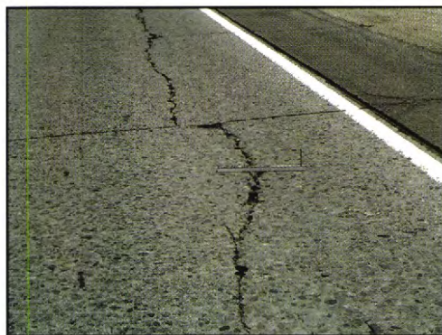
FIGURE 57 Distress Type JCP 3—High Severity Longitudinal Cracking
