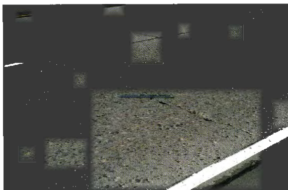
FIGURE 60 Distress Type JCP 4—High Severity Transverse Cracking
