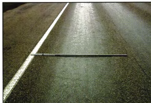
FIGURE 32 Distress Type ACP 9—Rutting
