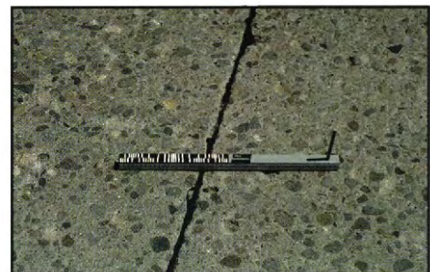
FIGURE 62 Distress Type JCP 5—Moderate Severity Joint Seal Damage
