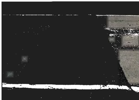
FIGURE 87 Distress Type JCP 15—Large, High Severity Asphalt Concrete Patch
