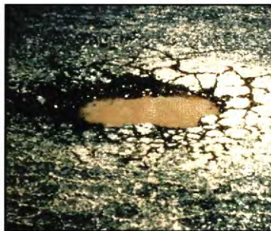
FIGURE 30 Distress Type ACP 8—High Severity Pothole, Close-up View
