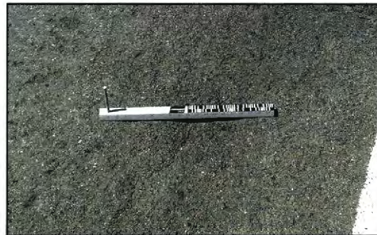
FIGURE 40 Distress Type ACP 13—Loss of Fine Aggregate
