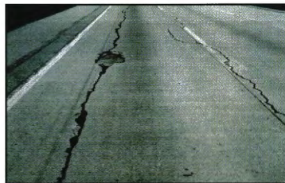
FIGURE 95 Distress Type CRCP 2—High Severity Longitudinal Cracking
