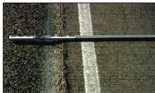
FIGURE 80 Distress Type JCP 13— Lane-to-Shoulder Dropoff
