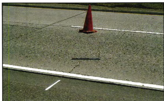
FIGURE 59 Distress Type JCP 4—Moderate Severity Transverse Cracking
