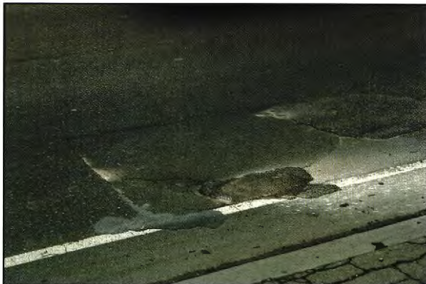
FIGURE 25 Distress Type ACP 7—High Severity Patch
