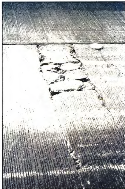
FIGURE 126 Distress Type CRCP 12—High Severity Punchout
