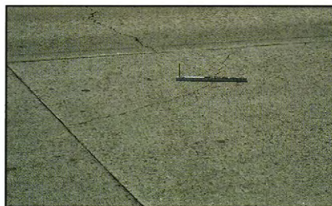
FIGURE 49 Distress Type JCP 1—Low Severity Corner Break
