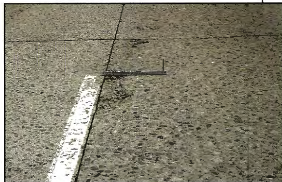
FIGURE 65 Distress Type JCP 6—High Severity Spalling of Longitudinal Joint
