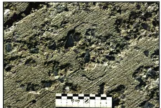
FIGURE 71 Distress Type JCP 8b—Scaling, Close-up View
