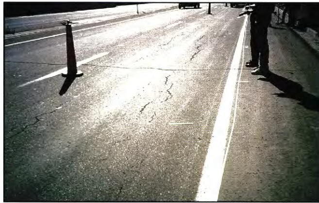
FIGURE 5 Distress Type ACP 1—Low Severity Fatigue Cracking
