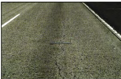
Figure 94 Distress Type CRCP 2—Low Severity Longitudinal Cracking
