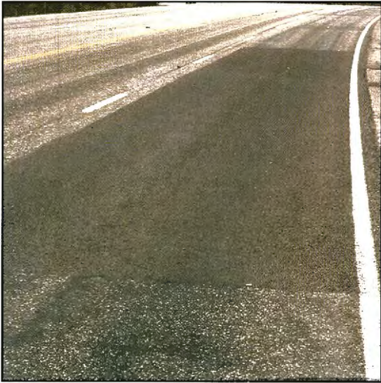
FIGURE 23 Distress Type ACP 7—Low Severity Patch
