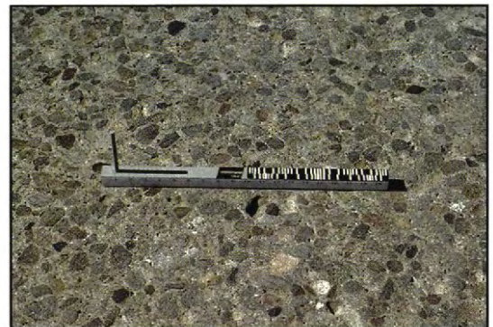
FIGURE 74 Distress Type JCP 10—A Popout
