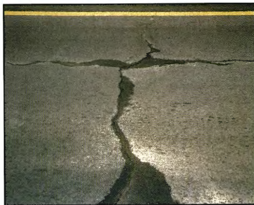
FIGURE 45 Distress Type ACP 15—Water Bleeding and Pumping
