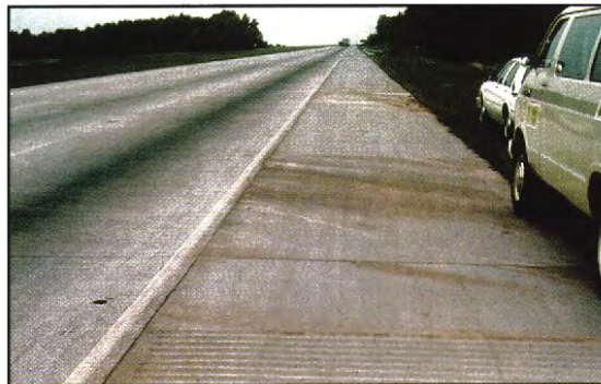
FIGURE 131 Distress Type CRCP 14—Water Bleeding and Pumping
