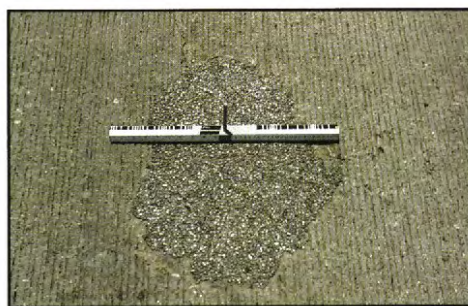
FIGURE 119 Distress Type CRCP 11—Small, Low Severity Asphalt Concrete Patch
