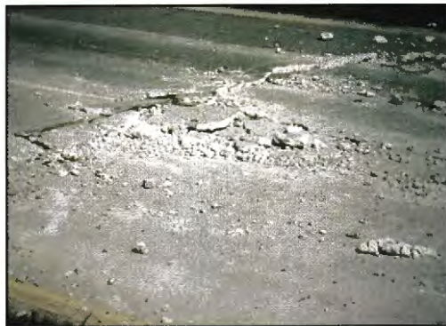
FIGURE 107 Distress Type CRCP 7—A Blowup
