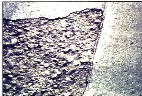
FIGURE 70 Distress Type JCP 8b—Scaling
