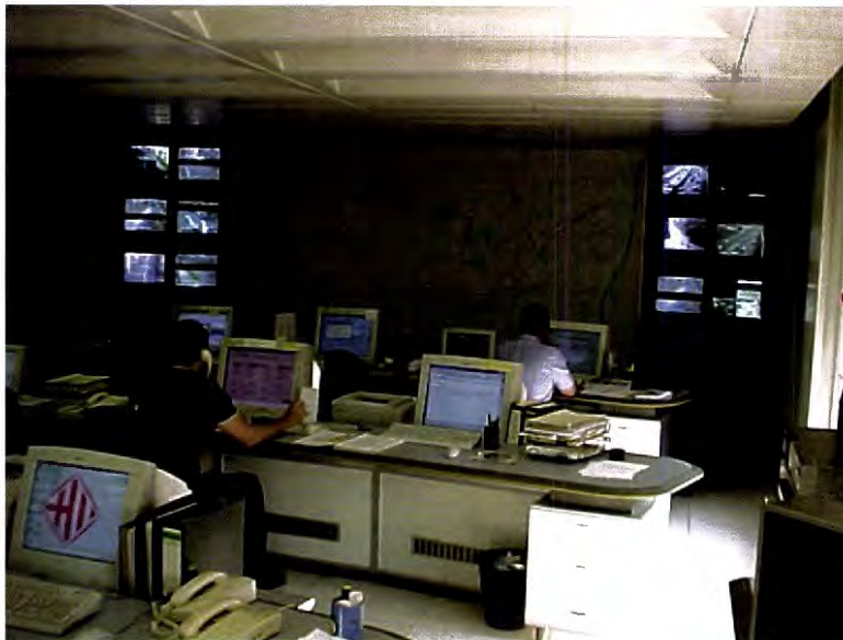
Figure 11. Barcelona City traffic management center.
