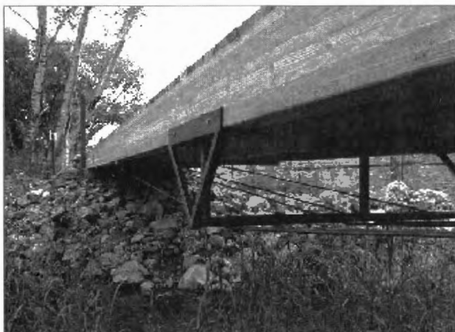
The Miller Creek permanent bridge tension frame was used to steady the bridge for pedestrians and bicyclists
