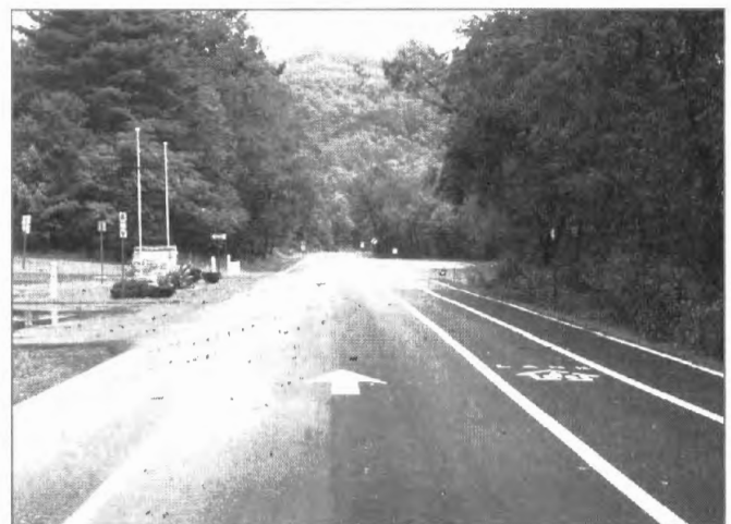
Striping of three travelways—center lane for one-way vehicle flow, a parallel flow bicycle lane on the right, and a contra-flow bicycle lane on the left.
