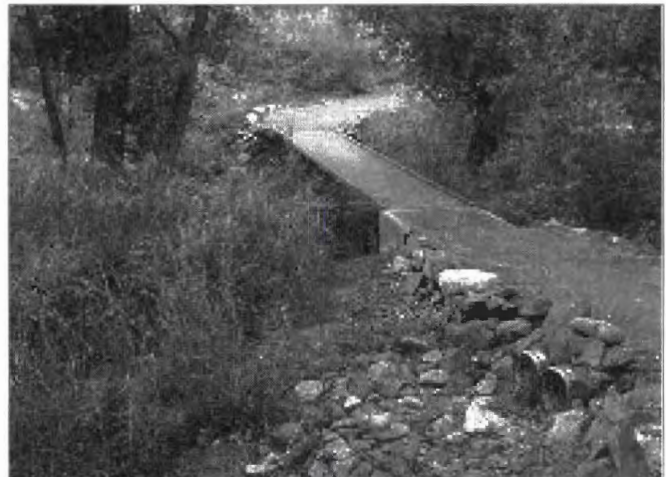
The Granite Creek bridge takes advantage of an existing sewer pipe as its foundation.
