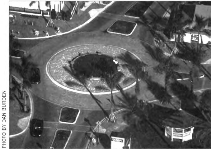
This Fort Pierce, Florida, roundabout is being constructed to reduce speeding, improve safety, and enhance the aesthetics of the community.
