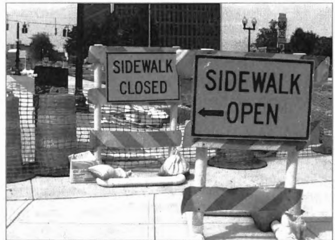
“Sidewalk Closed” and “Sidewalk Open” (with direction arrow) signs were posted on N. Pearl Street.
