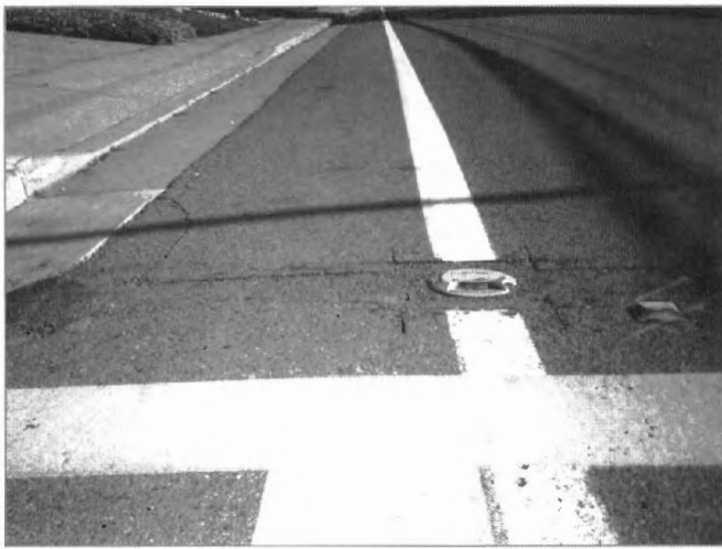
In-pavement lighting at crosswalk
