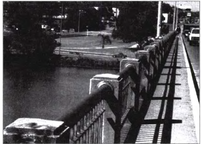
The sidewalk on the congested Lamar Bridge was only 1.1 m (3.5 ft) wide. Photo provided by the City of Austin.
