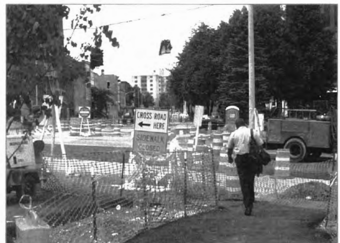
ADA compliant channelization to a pedestrian crossing was provided at N. Pearl and Clinton Street.
