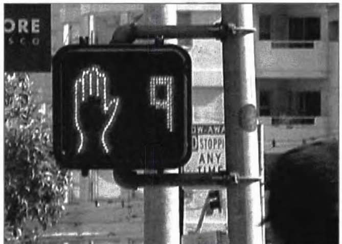
Pedestrian countdown signal heads show the time remaining for each phase.
