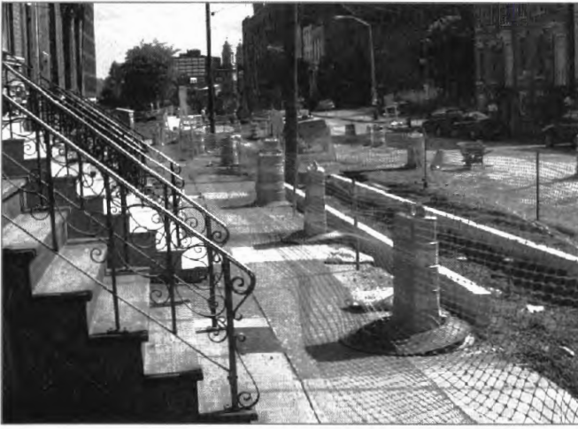
Cane-detectable fences were installed beside sidewalk widening and new curb work on N. Pearl Street.
