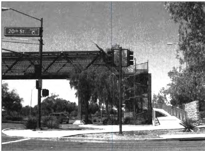
New ramps, spiral staircases, and footings were constructed to comply with ADA standards.
