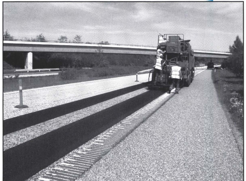
Figure 4. Replacing hot-mix asphalt in wheel paths in Denmark. (Photo source: Danish Road Institute, Denmark)
