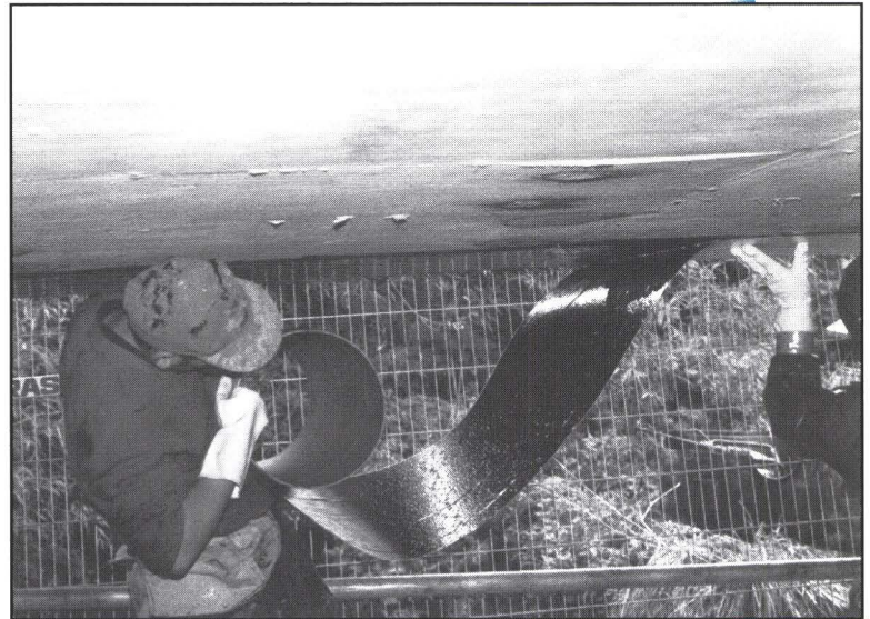
Figure 3. Fiber-reinforced strengthening of structures in the United Kingdom. (Photo source: TRL Limited, UK)
