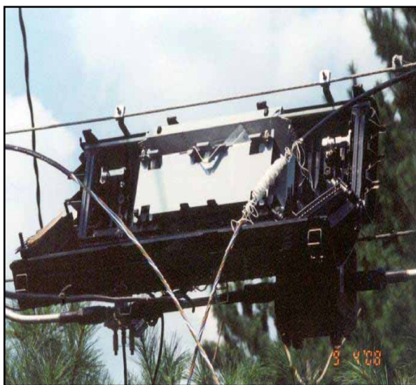
Figure 8-4: Aerial Fiber Optic Cable Splice Box - Photograph Courtesy Adesta, LLC
