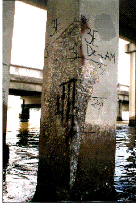
Figure 1.1. Photo. Cracked and spalled marine bridge piling.
