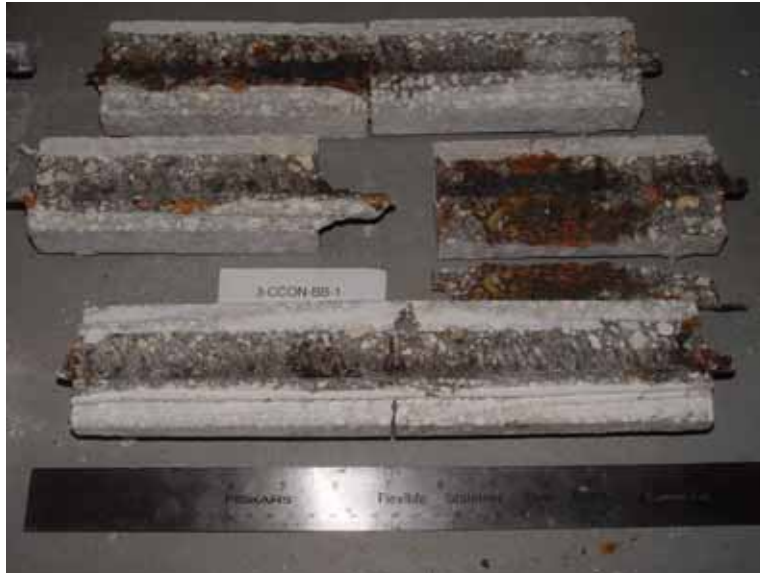
Figure 4.38. Photo. Traces of the upper three rebars and heavy corrosion products (specimen number 3-CCON-BB-1).
