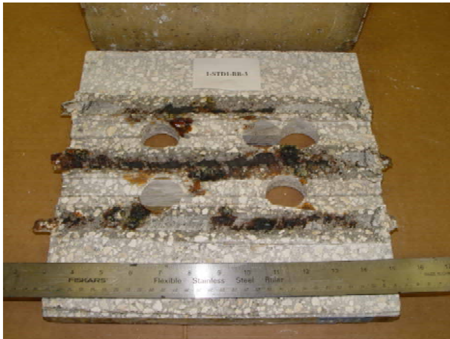
Figure 4.39. Photo. Trace of the upper rebars and heavy corrosion products on specimen number 1-STD1-BB-3.
