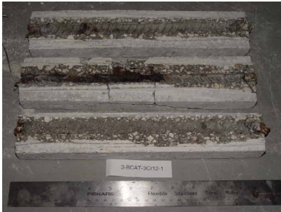
Figure 4.86. Photo. Trace of the upper rebar and corrosion products on specimen number 1-BCAT-3Cr12-1.
