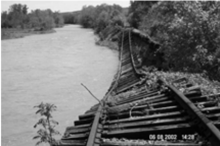
Southern Tier Line Washout – Before and After
