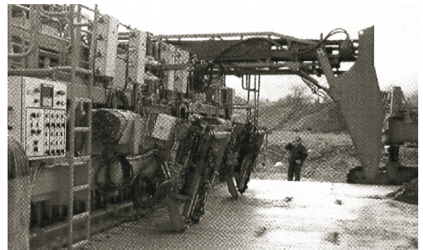
Figure 29. Dowel and tie bar inserters on back of front paver for two-lift paving in Austria.
