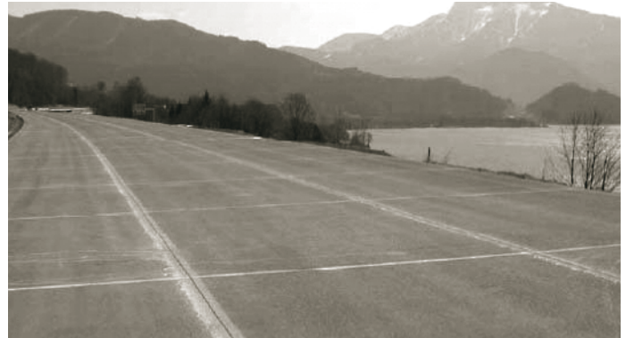
Figure 6. The A1 motorway in Austria, reconstructed in 2003 after more than 50 years of service.
