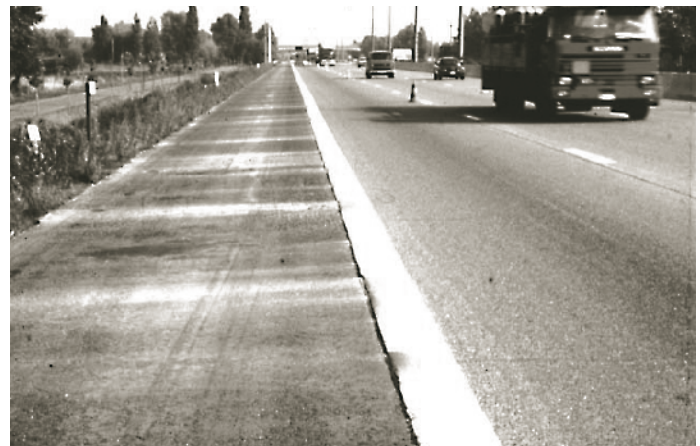
Figure 26. Pumping of fines from lean concrete base under Belgian CRCP built between 1977 and 1991.
