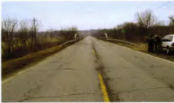
Buck Creek bridge (planned improvements include repaving, bridge improvements, and 8' paved shoulders)
