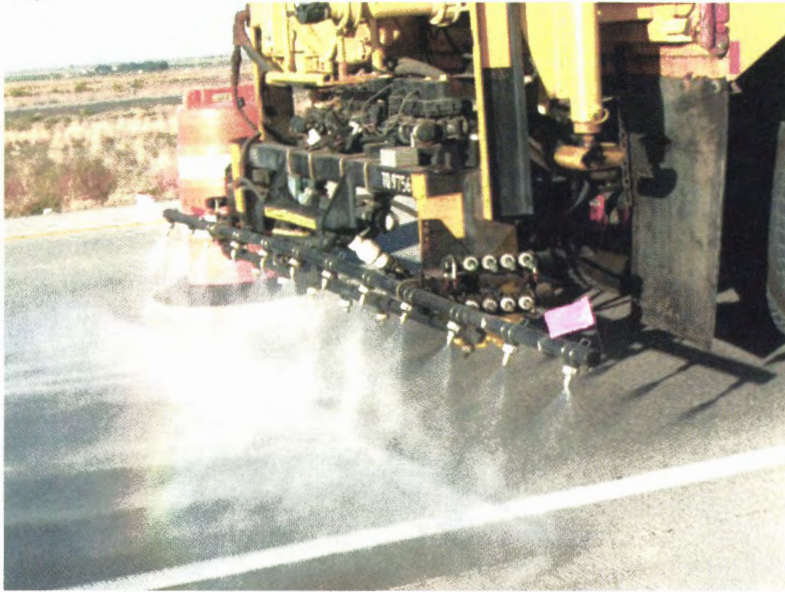
Figure 20. Spraying 30 percent \text{LiNO}_3 solution with a tanker truck on a concrete pavement near Mountain Home, ID.
