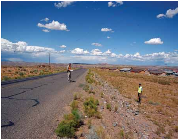
N-35 IN RED MESA, UTAH. PHOTO SHOWS LIMITED PAVEMENT WIDTH, LACK OF DELINEATION, AND CLOSE PROXIMITY OF ROADSIDE HAZARDS.
