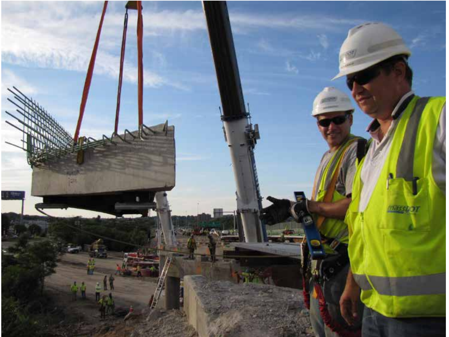
MassDOT construction inspector Alex Normandin and Assistant Resident Engineer Bob Blackmar on August 13, 2011, as one of the 94 Fast 14s 252 Prefabricated Bridge Units is lowered into place. MassDOT used this innovative method of construction to maximize mobility while safely replacing fourteen Boston-area bridges in just 10 weekends. Photo courtesy of Massachusetts DOT. Photographer: Eliza Partington.
