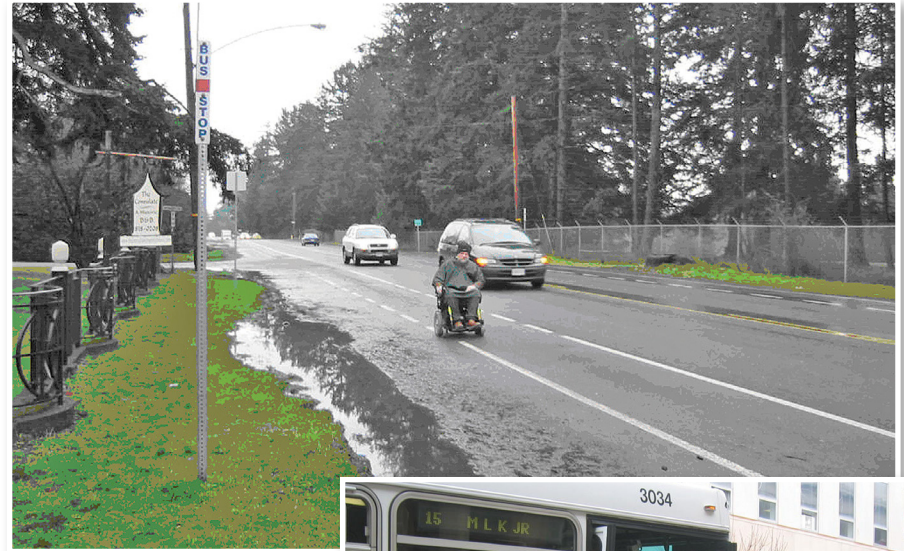
Above: The lack of a firm, stable and slip resistant boarding and alighting area and accessible connecting pathway makes this stop in British Columbia inaccessible. Rider safety is compromised as the poor drainage and grassy/muddy waiting area create slippery conditions. Source: BC Transit in British Columbia, Canada
