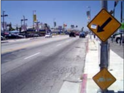
Rough pavement on Lankershim Boulevard, looking north from Killion Street
