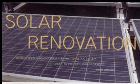
The PV array covers more than 62,000 square feet of space.
