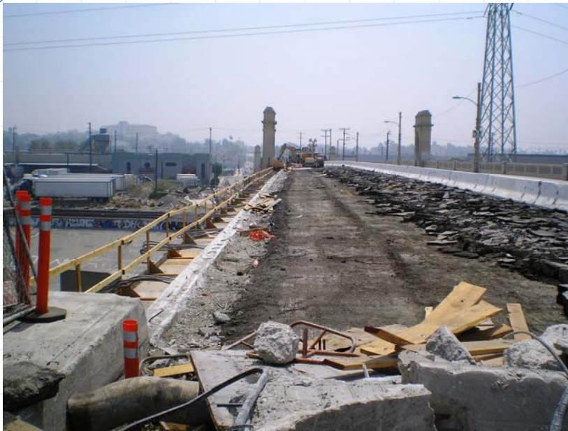
Parapet guardrail walls and paving along the north side of the bridge have been removed
