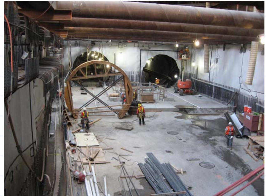
The excavation support struts are removed after the walls are poured and the concrete strengthens
