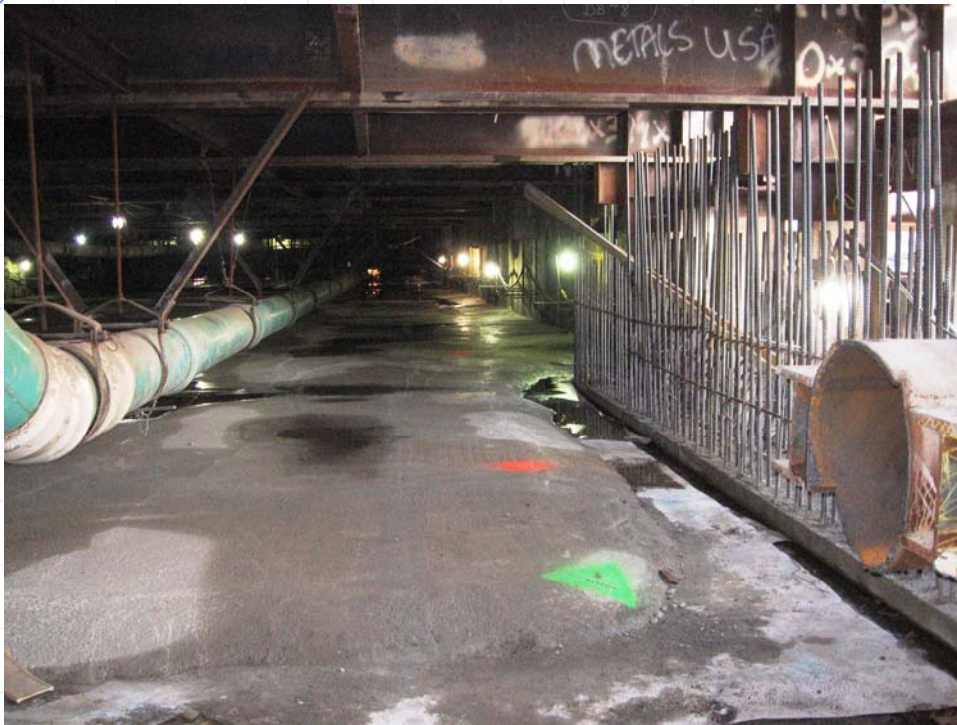
Boyle Heights/Mariachi Plaza Station roof slab construction has been completed. Surface exits and vent shafts are being constructed prior to removal of temporary concrete street deck.
