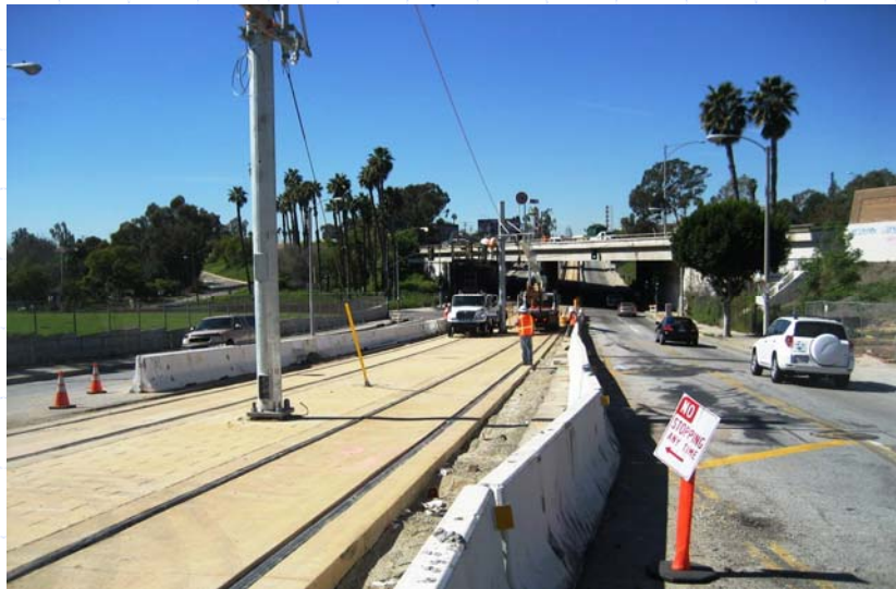
View west along 3 rd towards Downey near the 60 Freeway at the U-Channel.
