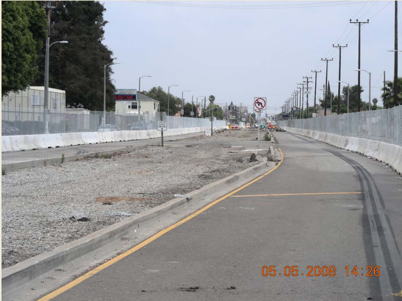
Installation of Chain Link Fence on K-rail along Exposition Blvd, between Vermont and 7th
