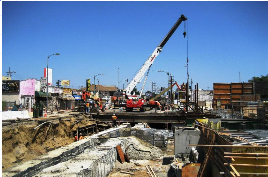
Concrete deck panels and steel deck beam removal over the 1 st /Soto underground station.
