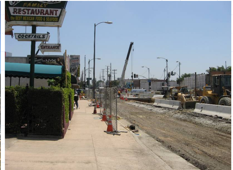
New colored sidewalks were installed before street demolition and deck removal to maintain pedestrian access.
